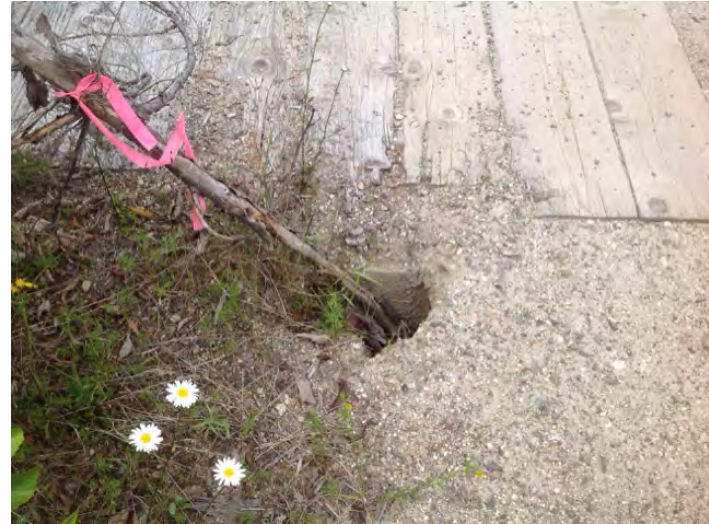
failing fill on right approach
