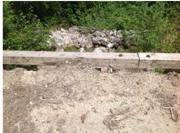
guardrail too low
